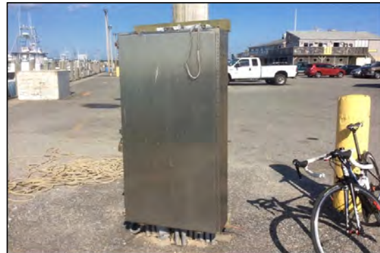
Flood proof utilities
