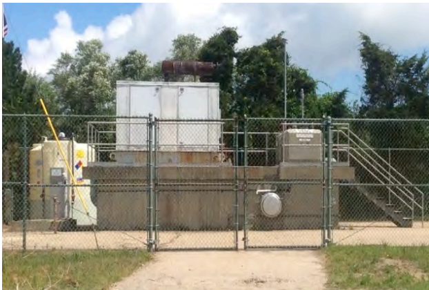
Elevated Utilities and Generator (Pt. Judith, RI)
