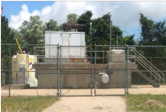
Elevate Utilities and Generator
