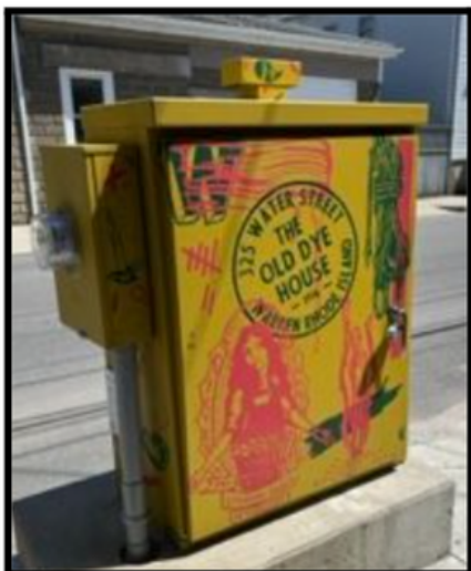
Electric Box on Water Street
