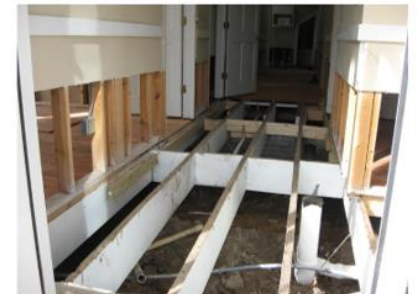
An example of flood proofing is the addition of pumps into the basement of the building at 901-903 Front Street as well as adding water-resistant flooring on the ground floor.
