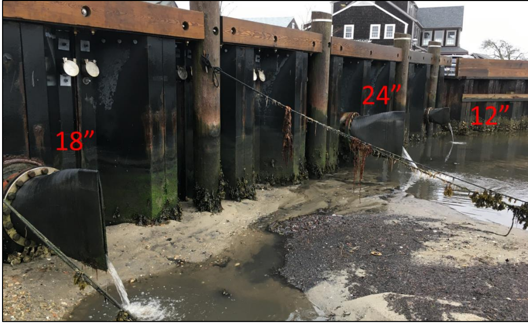
Figure 13, Storm Water Outfalls and Check Valves at the Easy Street Bulkhead (2/13/2020) 8
