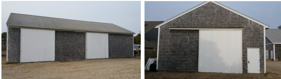
Photo Gosnold center Annex Building – left existing south Elevation, right existing west elevation. Rehabilitating this existing shell storage building into usable heated space will be a major project.
