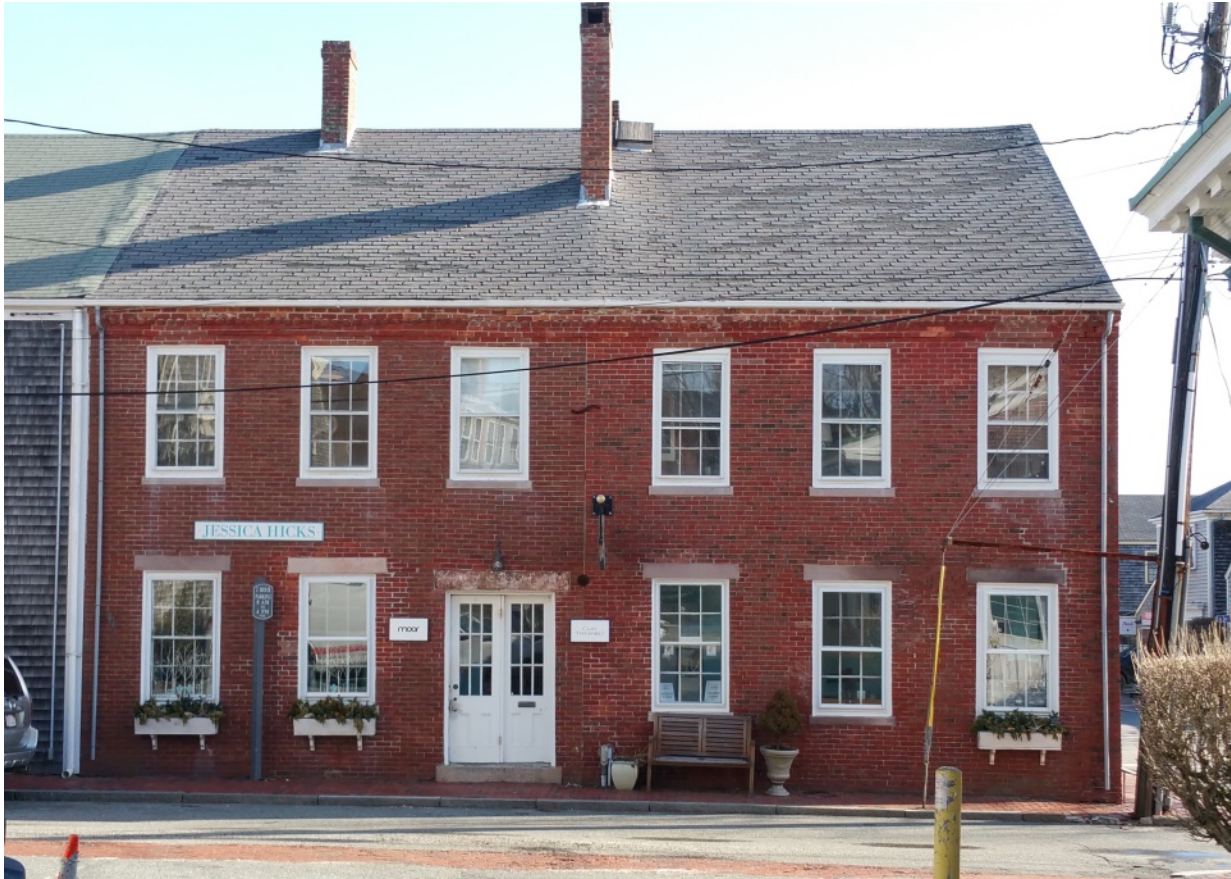
Photo of the West Elevation of #2 Union Street. Note the very poor condition of the asphalt roofing shingles. The roof hatch and chimney will also require repair. This work must be scheduled in the very near future.
