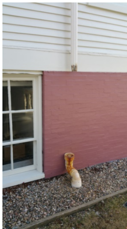
Photo East Elevation of the Hadwen House – all the downspouts along the perimeter of the Hadwen house must be immediately checked and re-connected to the subsurface storm water drains.
