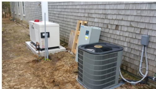
Gosnold Center Photo: A new 5KW emergency generator and a new condenser unit have recently been installed at the center
