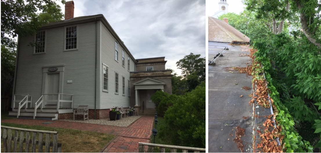
Photo of the Front Elevation of the Quaker Meeting House – Overhanging tree branches can damage a roof or gutters in a wind storm and leaf debris will clog gutters and downspouts.
