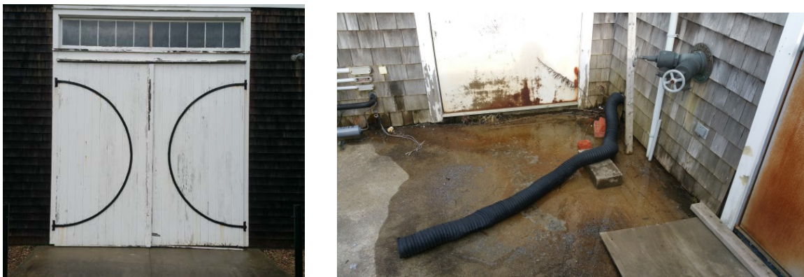
Gosnold Support Center: 2018 Task #1 Inset receiving room barn doors, install Plexiglas transom storm window, paint the front elevation doors and trim; Task #2 Install a drainage channel to carry chiller condensate drainage and fire pump drainage away from the corner of the building.
