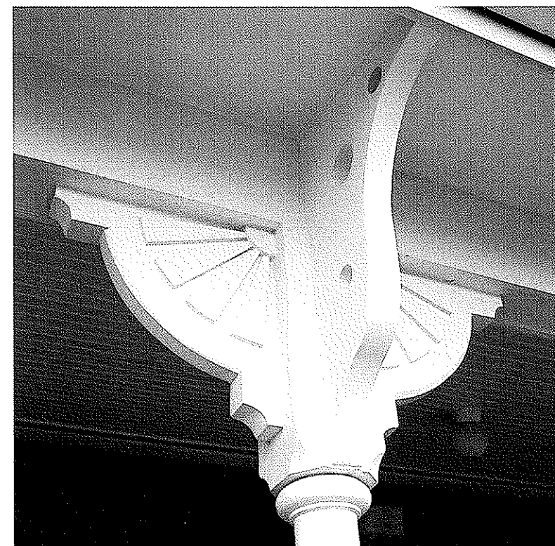
FIGURE 13: Detail of Sandanwede, Hulbert Avenue. Sandanwede is notable for its distinct sunburst-motif porch supports. The supports and trim were originally painted a warm, neutral color that complemented the facade and harmonized with nature. In the Victorian era white was considered too cold and glaring and was rarely used on exteriors.
