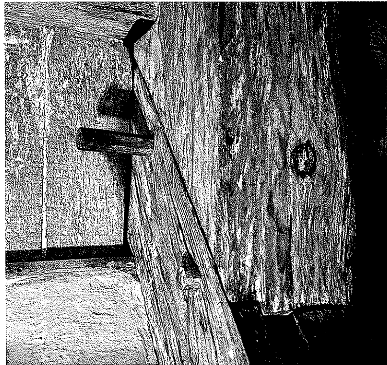
FIGURE B: Timber Frame Detail at the Captain Richard Gardner House, Built ca. 1722–24, 34 West Chester Street. Exposed timbers at the peak of the house reveal the trunnel (peg) that fastens together the mortise-and-tenon joint of a pair of roof timbers. The board planking used to sheath the building interior was usually whitewashed, and interior walls were given an additional layer of plaster for insulation and finish. On the exterior, the boarding was covered with an added layer of shingles.
