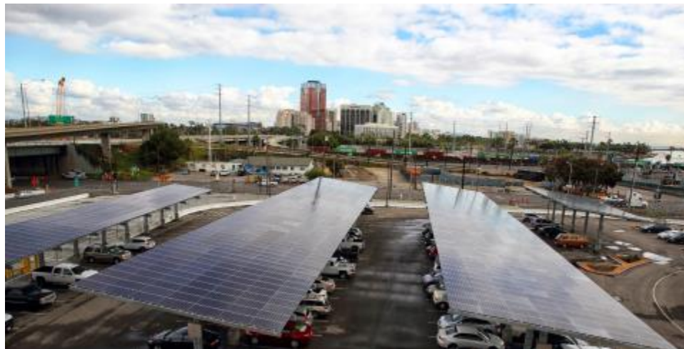
Figure 5: Port of Long Beach- Solar Photovoltaic (PV) System ( https://mms.businesswire.com/media/20161129005487/en/557318/5/2016-11-PFMG-LB-310-edited.jpg )
