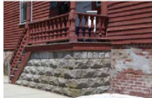
Inappropriate The material used for the stairs is not consistent with the foundation material.
