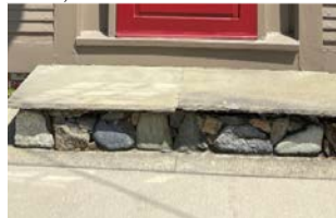
Inappropriate The material used for the stairs is not consistent with the foundation material.
